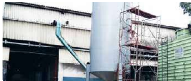
Commissioning of conical bottom 20KL vertical lubetank installation at institutional customer premises
