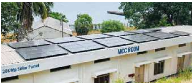
Completed solarisation of Trincomalee terminal with 20 KWP
