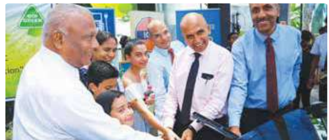
Installation of EV charging station at newly commissioned RO at Colombo making total 5 EV charging station at LIOC retail outlets across island
